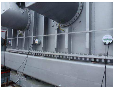
Figure 2: Sensing heads mounted on the transformer.
