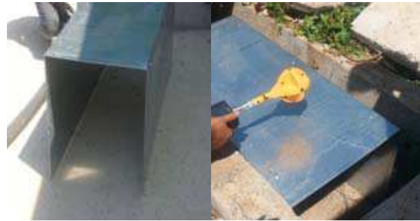
Figure 2: Measurement in the high voltage channel with reversed U galvanized shielding.
