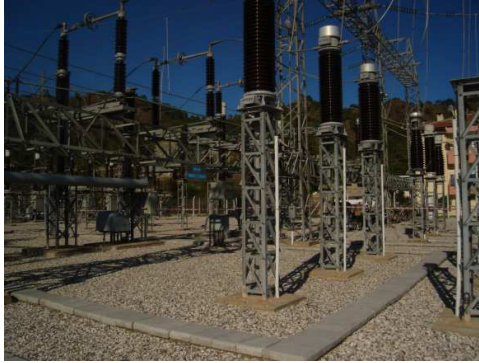
Figure 1: Open areas of the substation.
